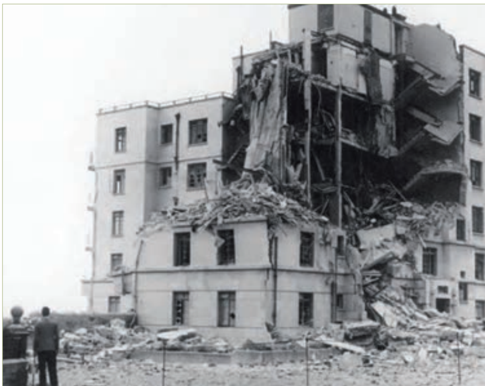
The damaged Suffolk House flats in Barrassey Road, Bexhill in East Sussex. Photo: © Author
