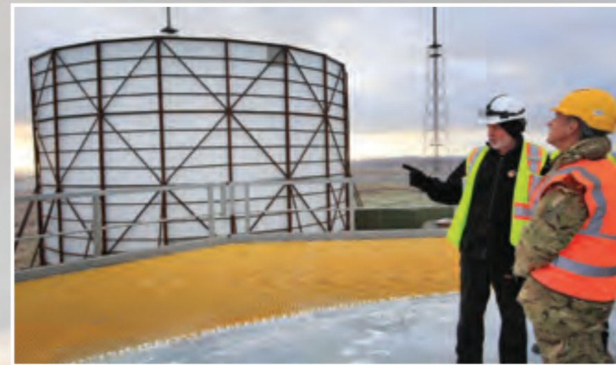
Left: Chief of the Air Staff, Air Chief Marshal Sir Stephen Hillier, (in yellow hard hat) is shown round the site for the new remote radar head at Saxa Vord, Unst, Shetland. © MOD/Crown
